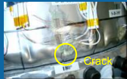
Crack (water leakage)
