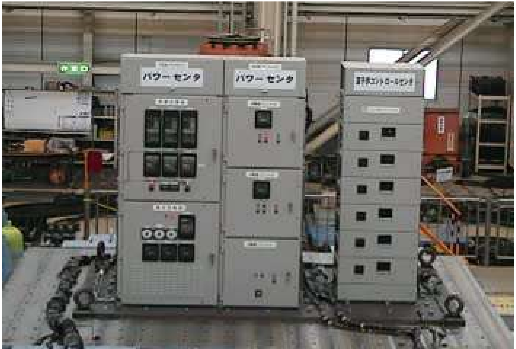
Power Center & Reactor Control Center (Maximum input acceleration = 6 \times 9.8 \text{m/s}^2 )
